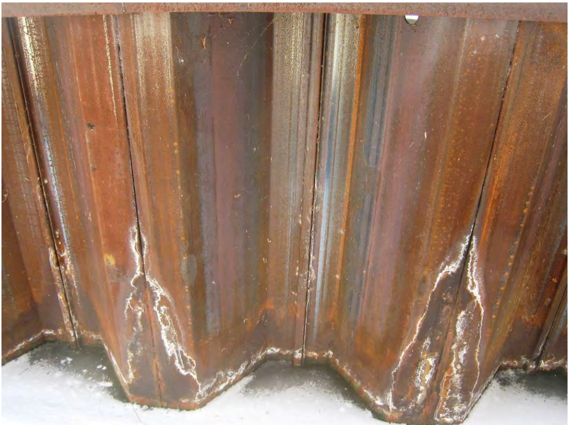
Photo 4 – Corrosion at Joints
