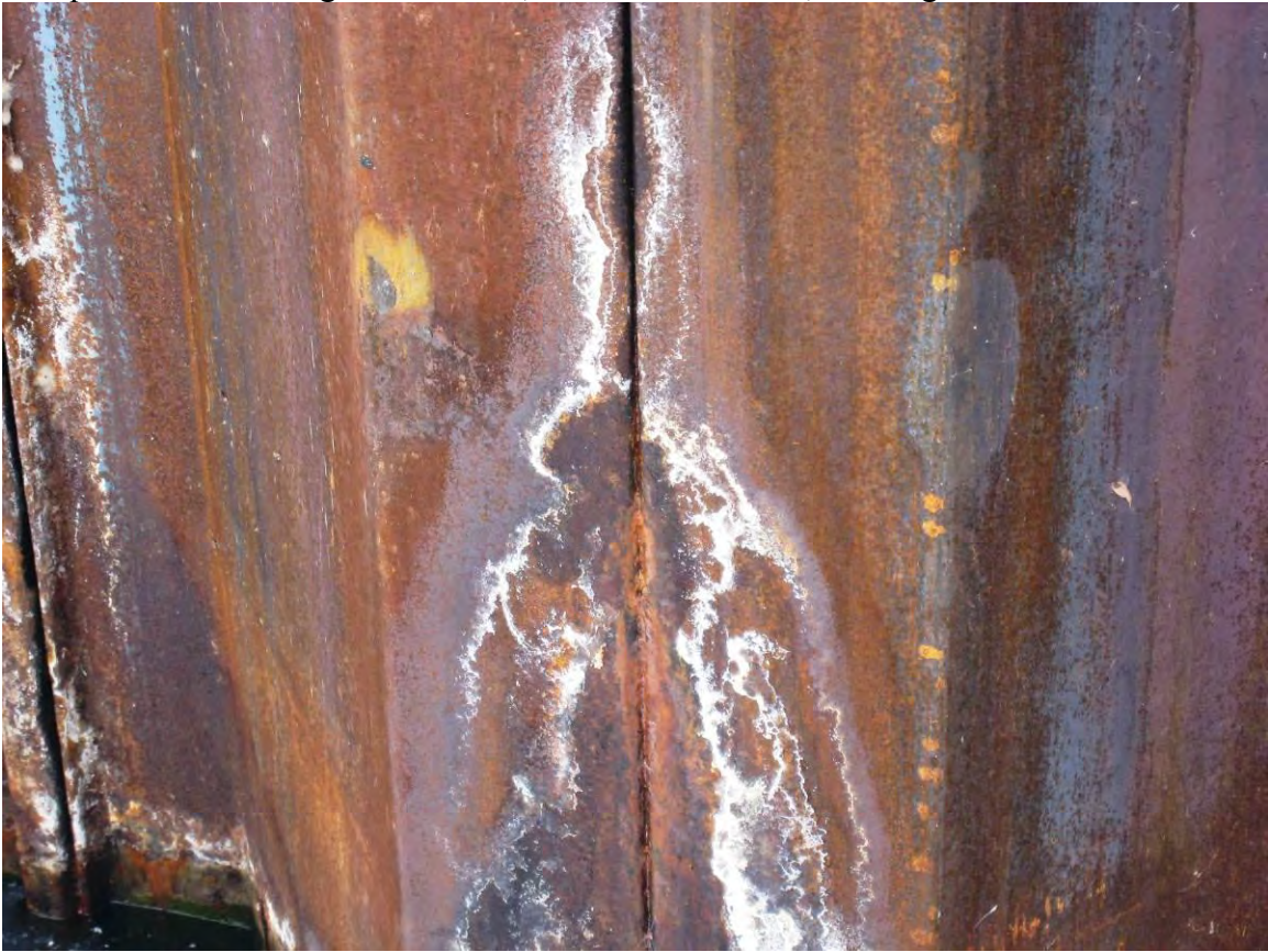
Photo 5 – Spot with Localized Corrosion
