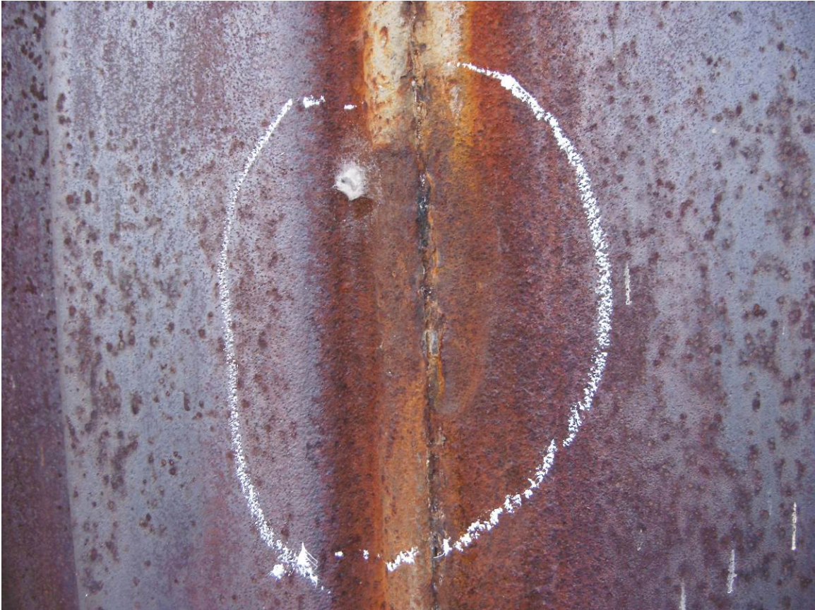
Photo 5 – Spot with Localized Corrosion
