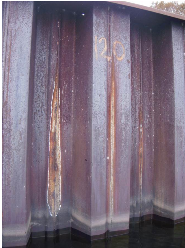
Photo 4 – Corrosion at Joints
