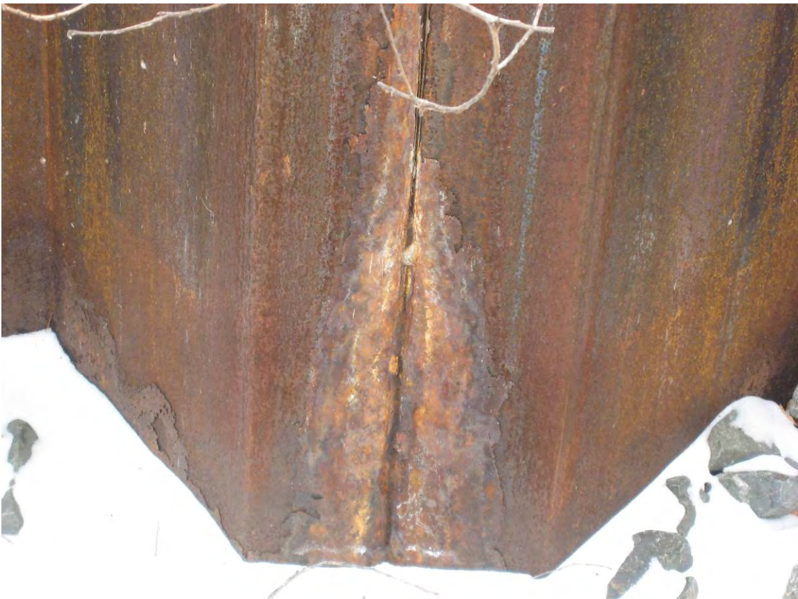
Photo 4 – Corrosion at Joints
