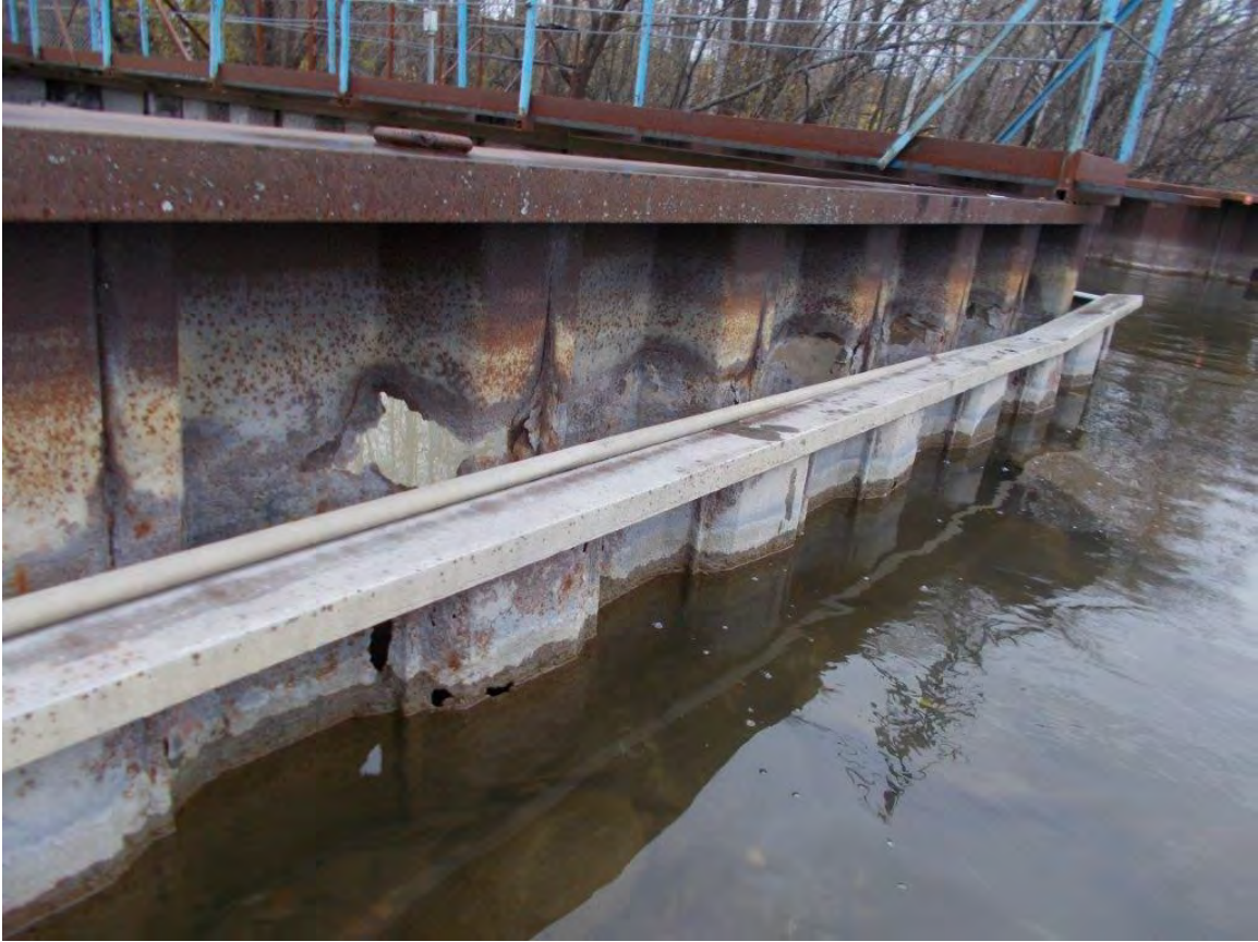
Photo 5 – Interior Walls in Poor Condition
