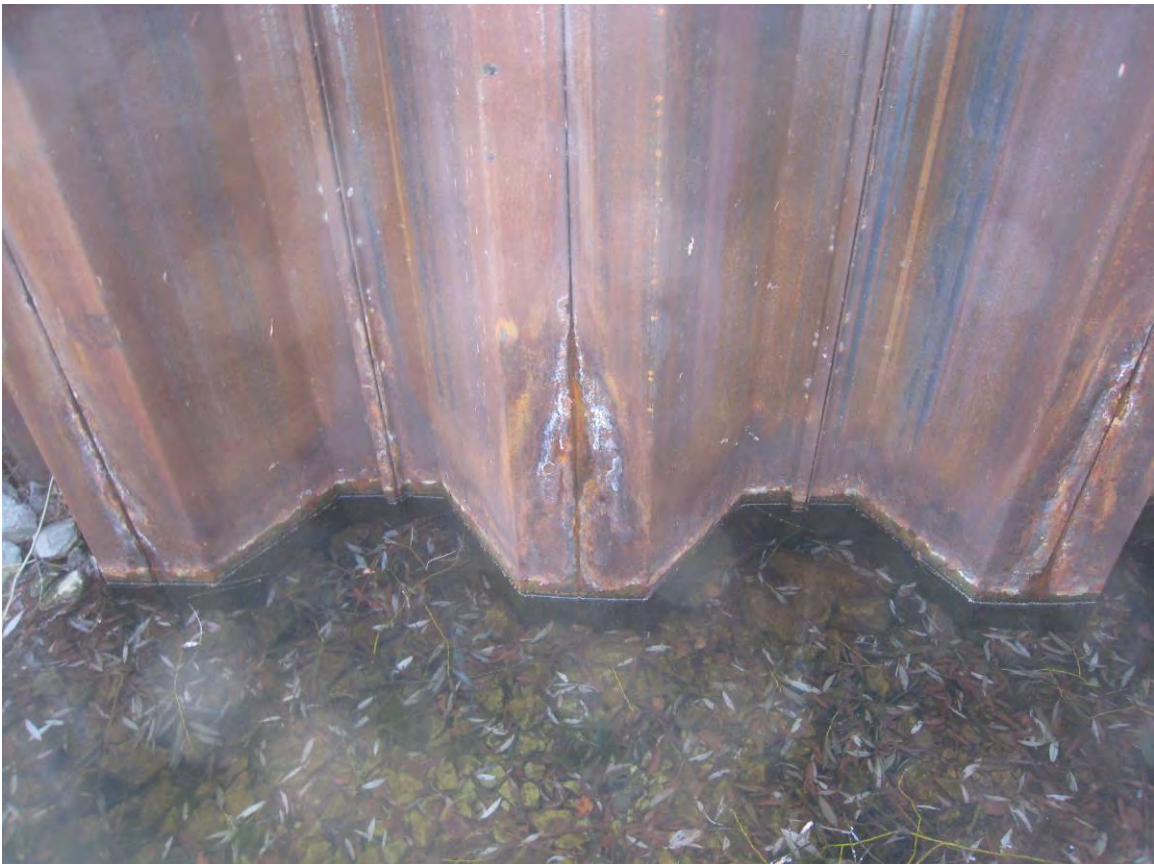
Photo 4 – Corrosion at Joints
