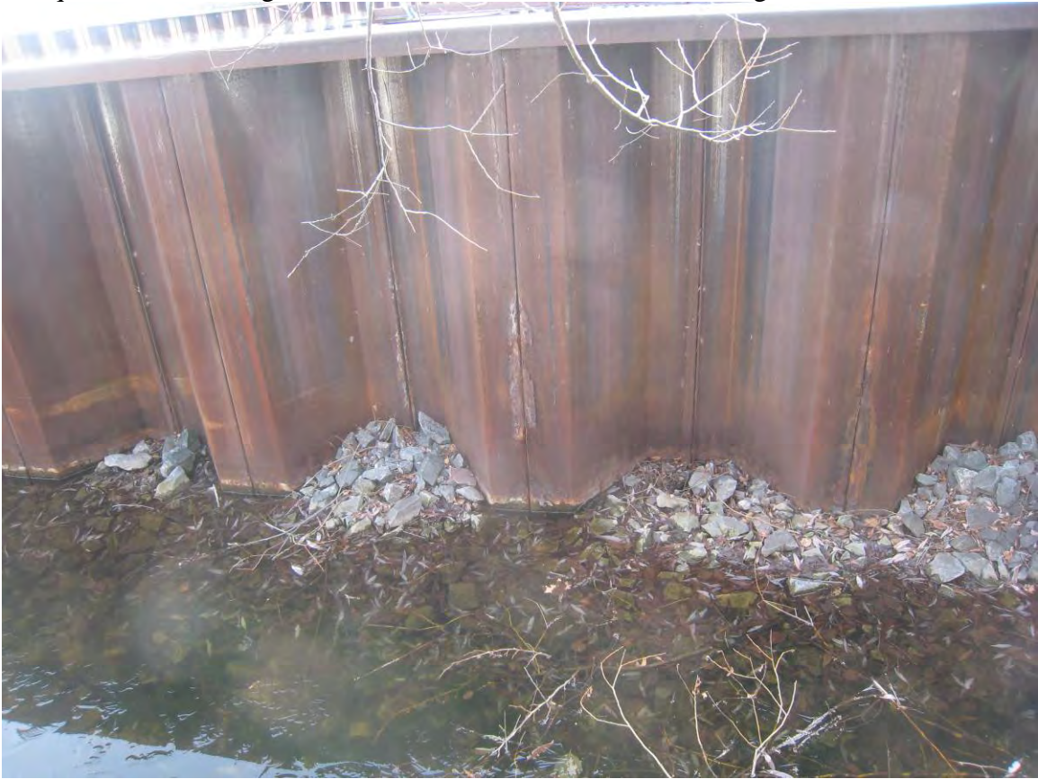
Photo 5 – Spot with Localized Corrosion
