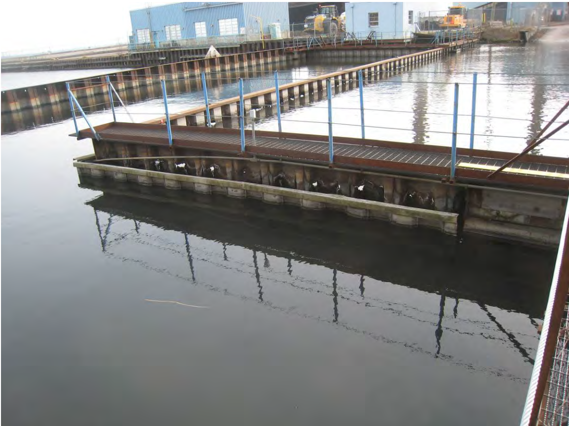
Photo 6 – Interior Walls in Poor Condition
