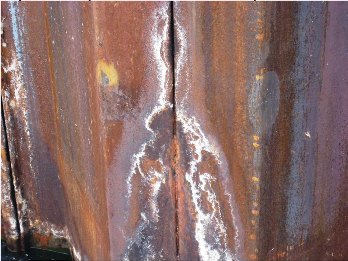
Photo 5 – Spot with Localized Corrosion
